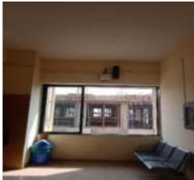
CCTV Camera [Corridor]
